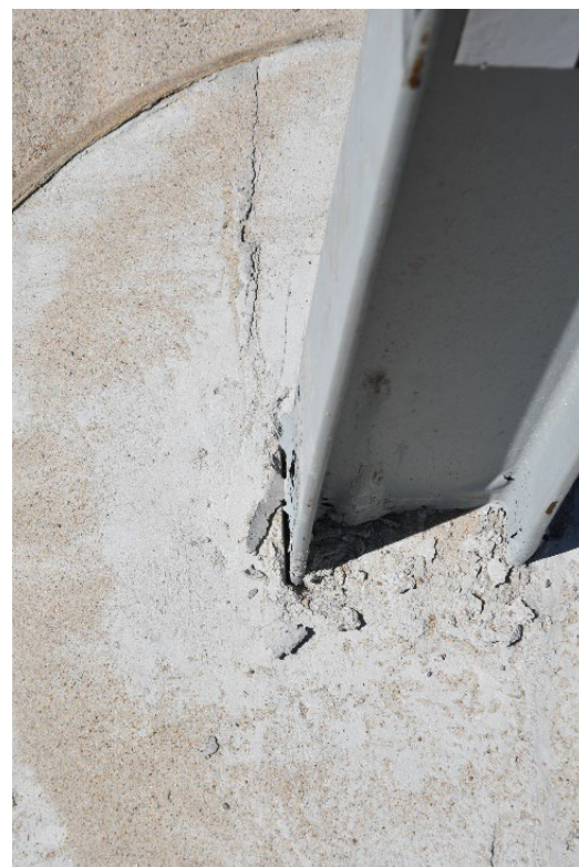
Figure 6.10 Additional Time-Sequential and Damage Photographs, Test No. AKLP-3
