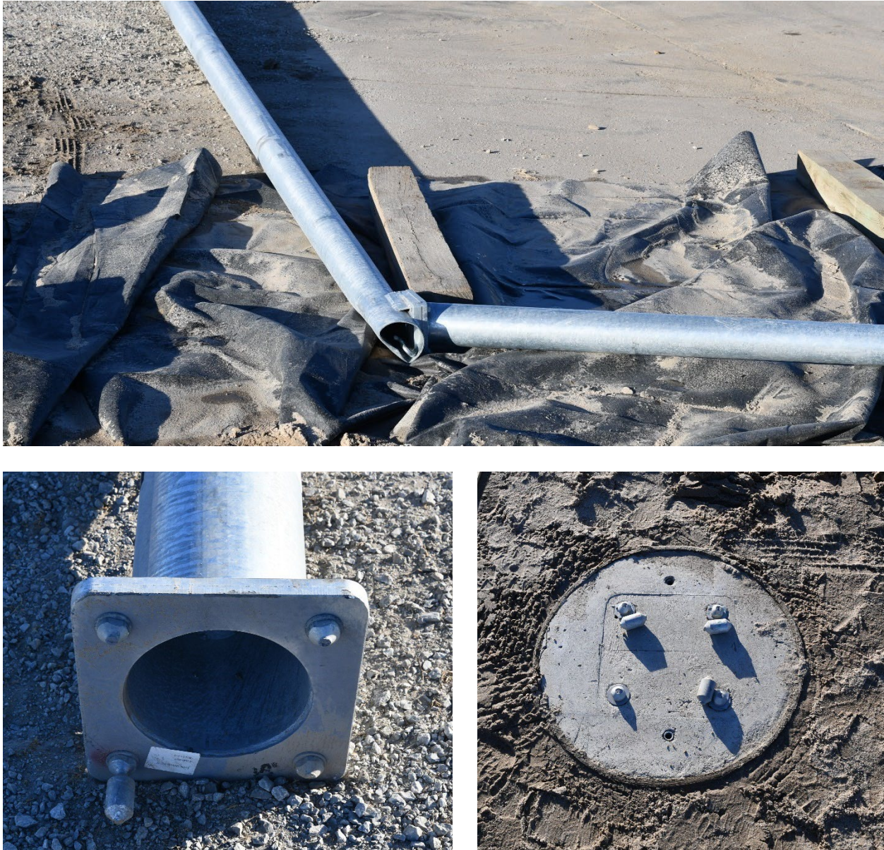
Figure 8.10 Additional System Damage Photographs, Test No. AKLP-6
