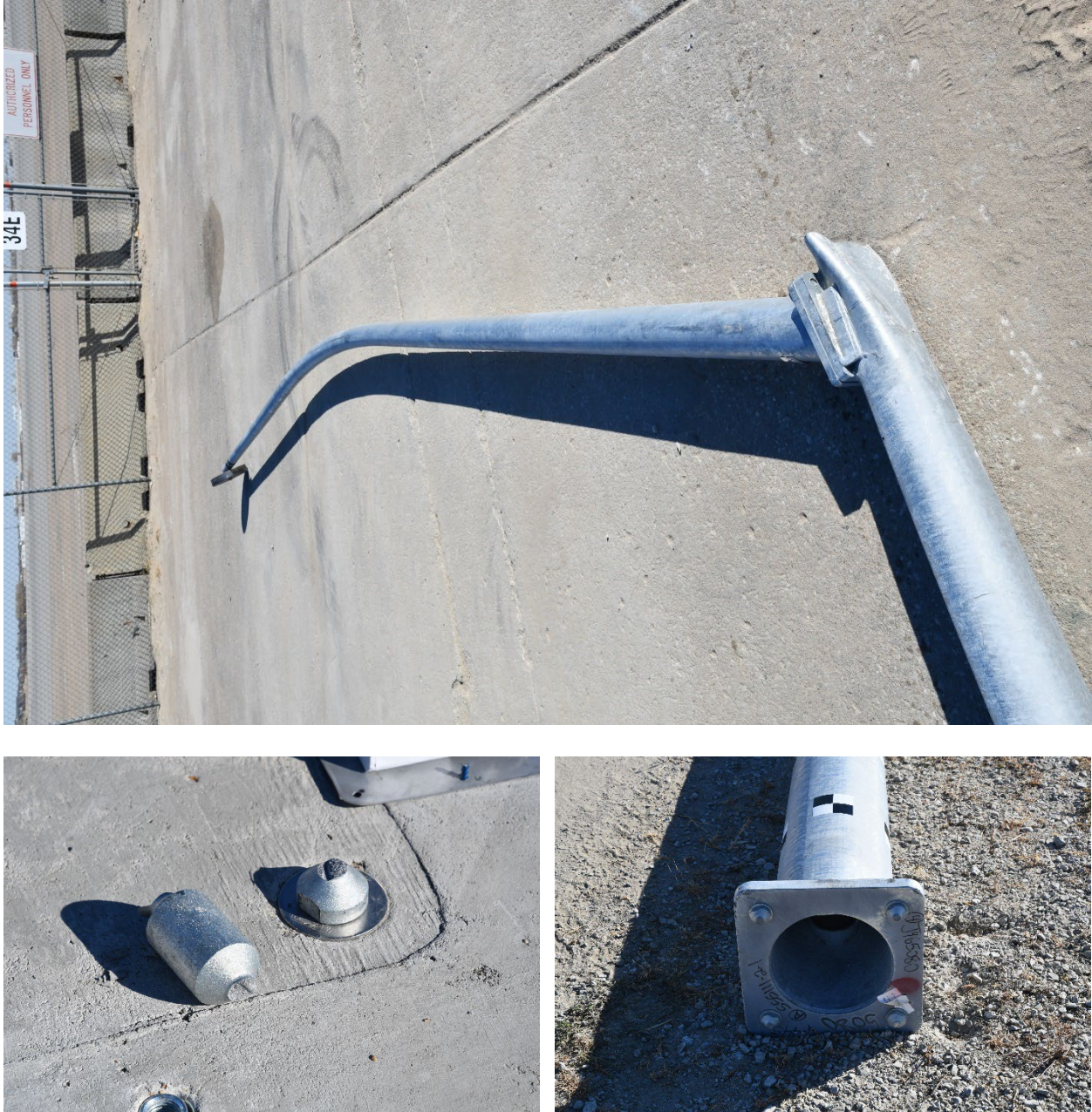
Figure 8.4 Additional System Damage Photographs, Test No. AKLP-5
