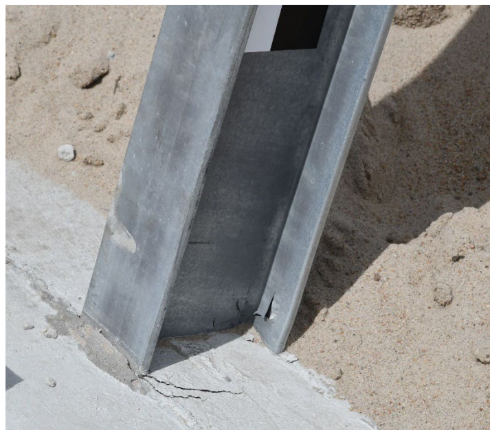
Figure 6.6 Additional Time-Sequential and Damage Photographs, Test No. AKLP-2
